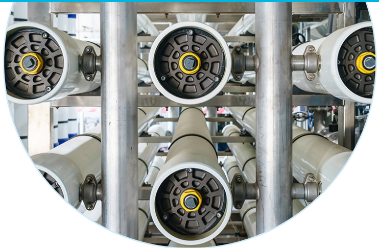
Filtration with reverse osmosis.
